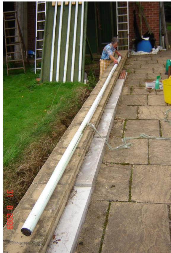
Pipe laid on low wall to make it easier to work on
